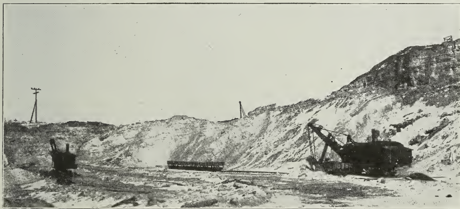
Fig. 31. Quarry of National Silica Company showing steam shovel used for loading sand, and cars which transport the sand to plant. (Photograph by courtesy of National Silica Company.)
